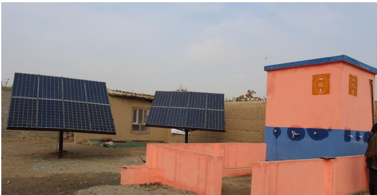
Figure 1: The SPW project is an environment friendly intervention providing needy communities with clean drinking water
